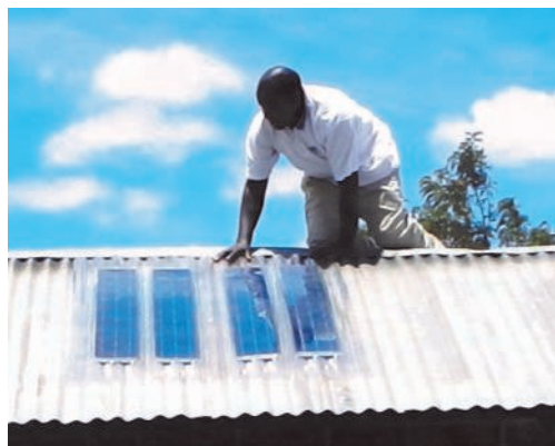
Picture: Solamander 135 Watt Photovoltaic Panel mounted on a corrugated roof
